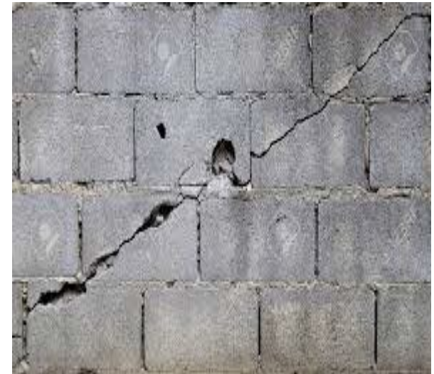
Cracks in wall surface
