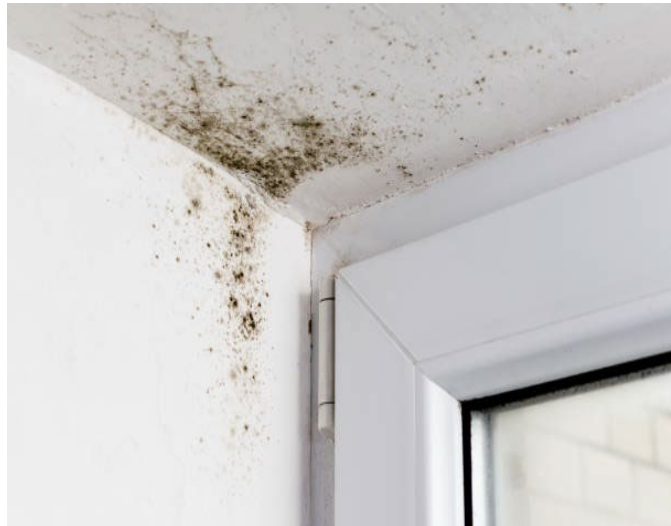
Mouldy Wall & Ceiling
